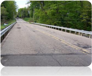
The above photo shows the existing condition of the West Spring Lake Road bridge over Cornelius Bayou.
